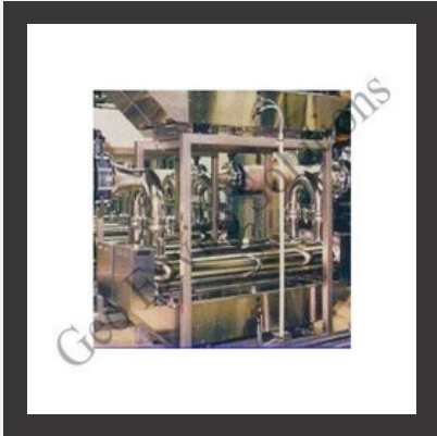
Iron Removal System
