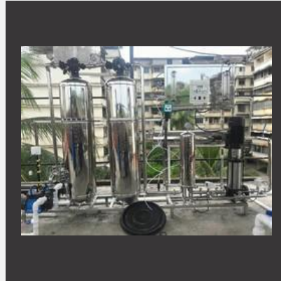
1000LPH RO Plant Fully SS
