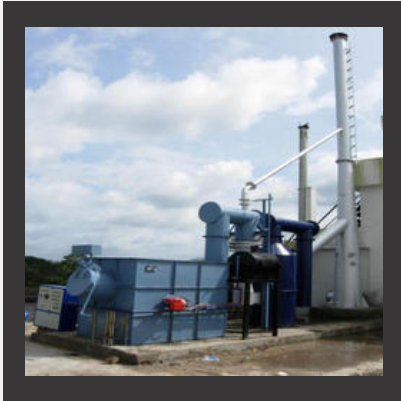
Bio Medical Waste Incinerator
